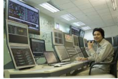
Pressure Control Room for NGV Stations
